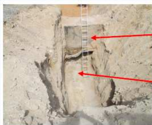
Concrete slab and unsafe access
