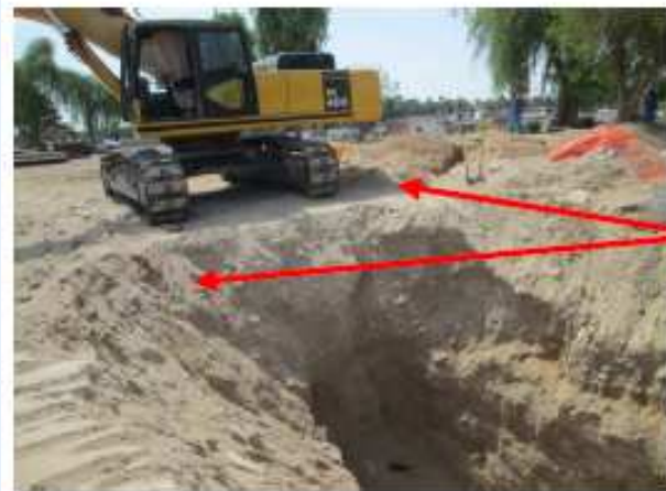
Absence of edge protection/bunding, stop blocks, signage and banksmen, stored spoil
